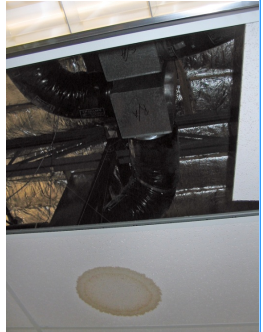
Interior view of leak under return air plenum
