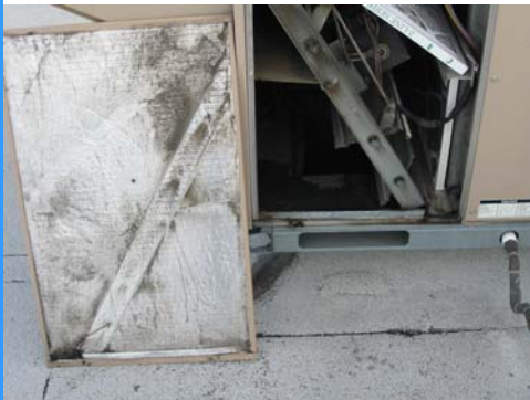
Filter access panel opened
