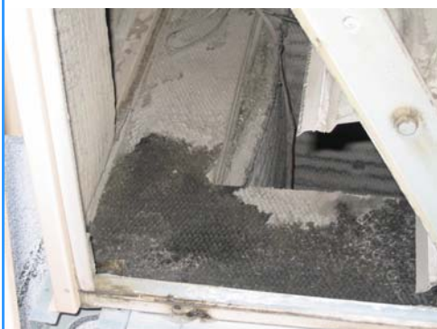
Water inside HVAC
