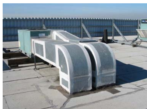
Side discharge with exposed ductwork
