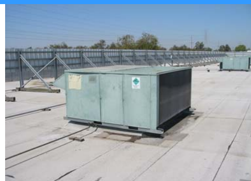
Bottom discharge-no exposed ductwork
